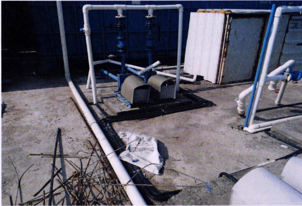
Fig. 4: Pumps for the sewage pipes
