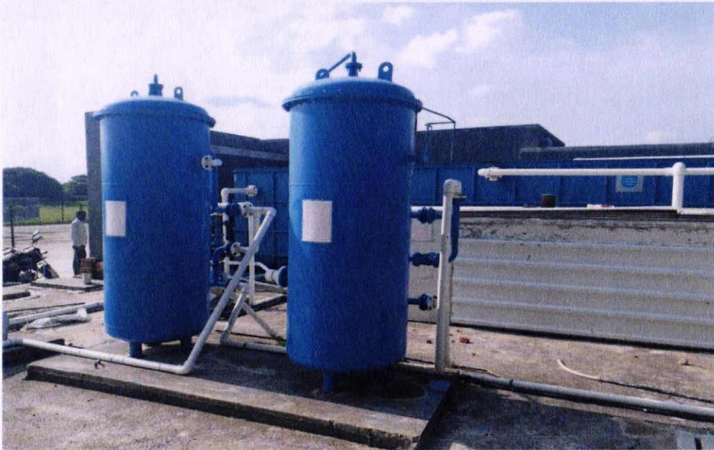
Fig. 5: Bioreactors installed in university
