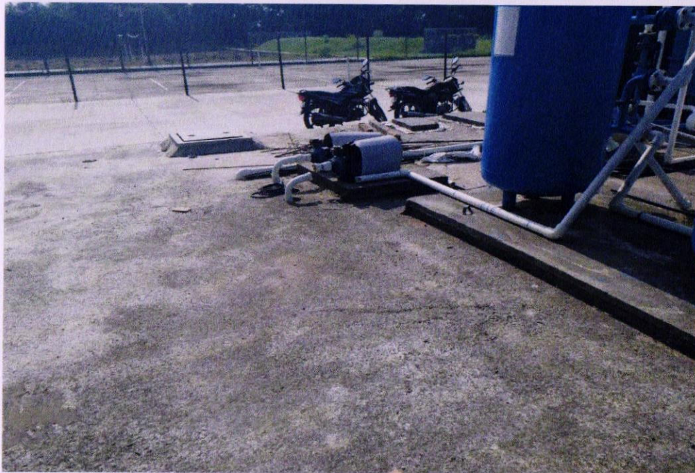
Fig. 2&3: Pipeline for sewage water
